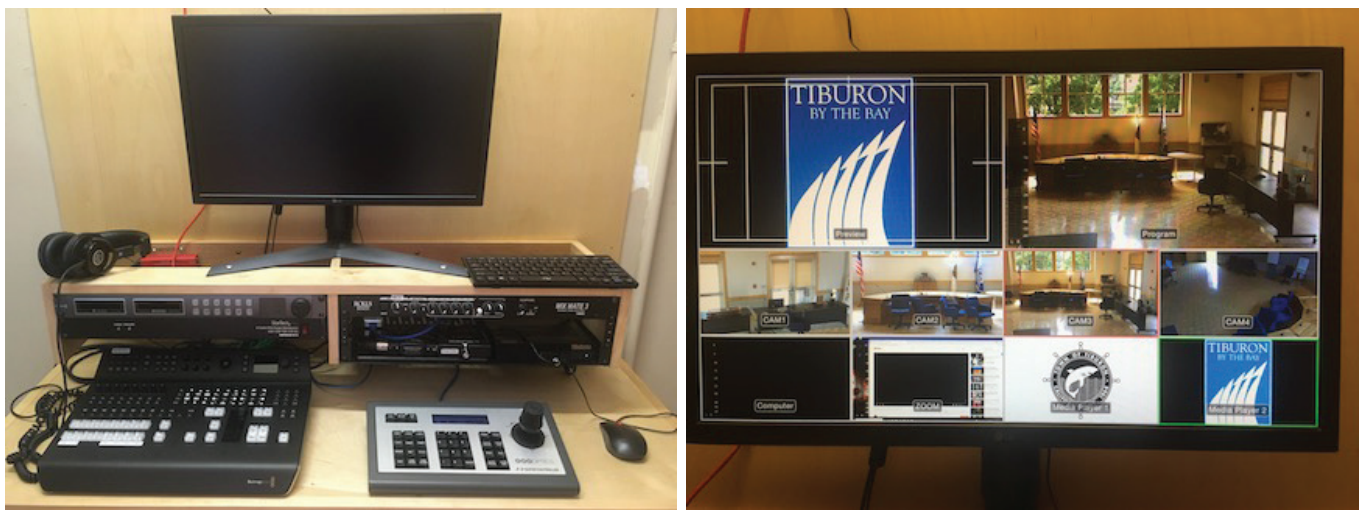
New four camera installation, this one in Tiburon is identical to other CMCM city installations.
